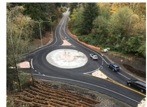
Crews finish new roundabouts on SR 524 at Locust and Larch ways View larger photos
